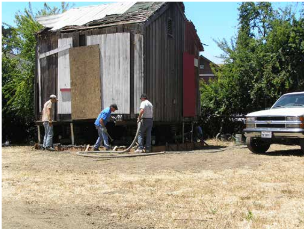
Cambria Chinese Temple Following its Relocation, Prior to its Placement on New Foundation Photo Taken July 6, 2007
