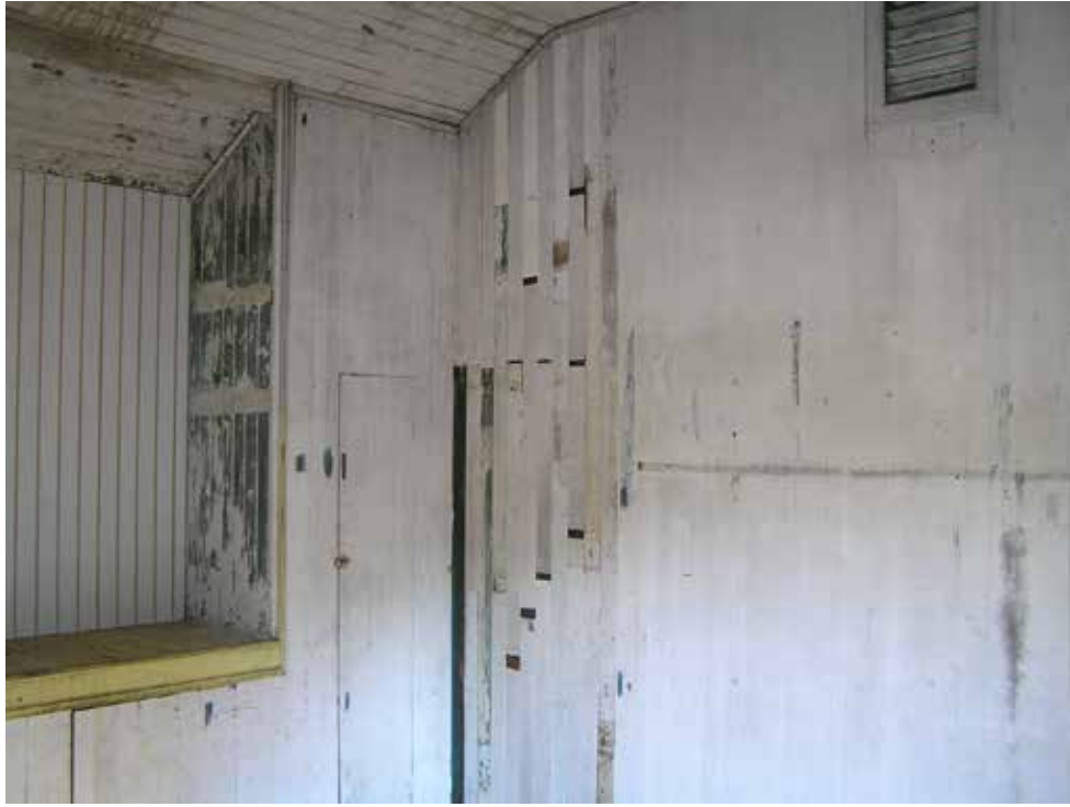
Interior View of Cambria Chinese Temple (North and West Walls) Following Wall Cladding Repairs and Prior to Paint Restoration Photo Taken Ca 2007
